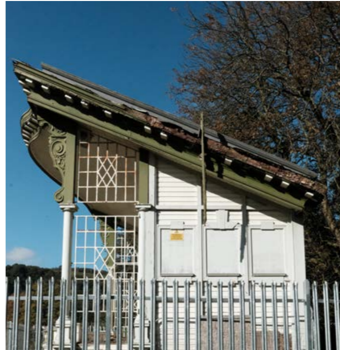
Damage and wet rot to the roof verge on the East Elevation
