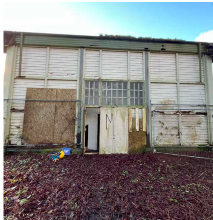
Rainwater downpipes missing and vegetation blocking gutter.
